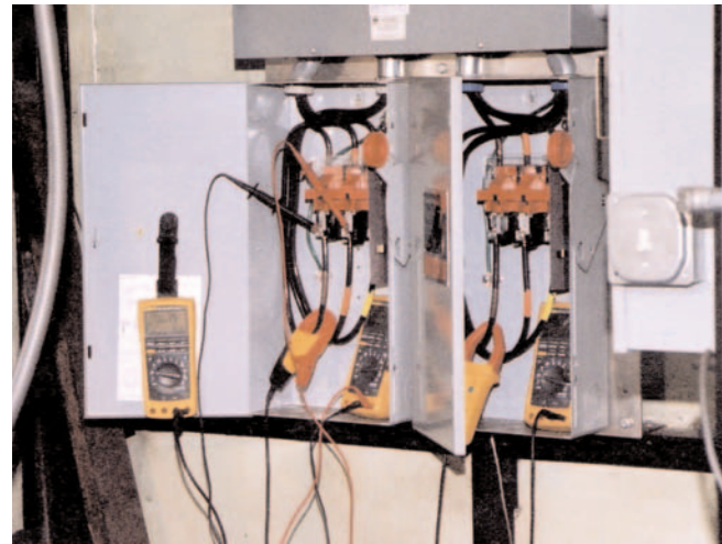
Simultaneous current and voltage logging at the control panel for two drive motors.
