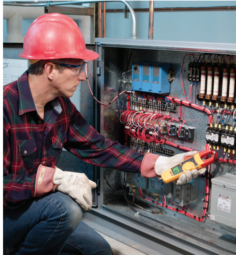
Checking current on a compressor controller with a true-rms Fluke 902 HVAC Clamp Meter.
